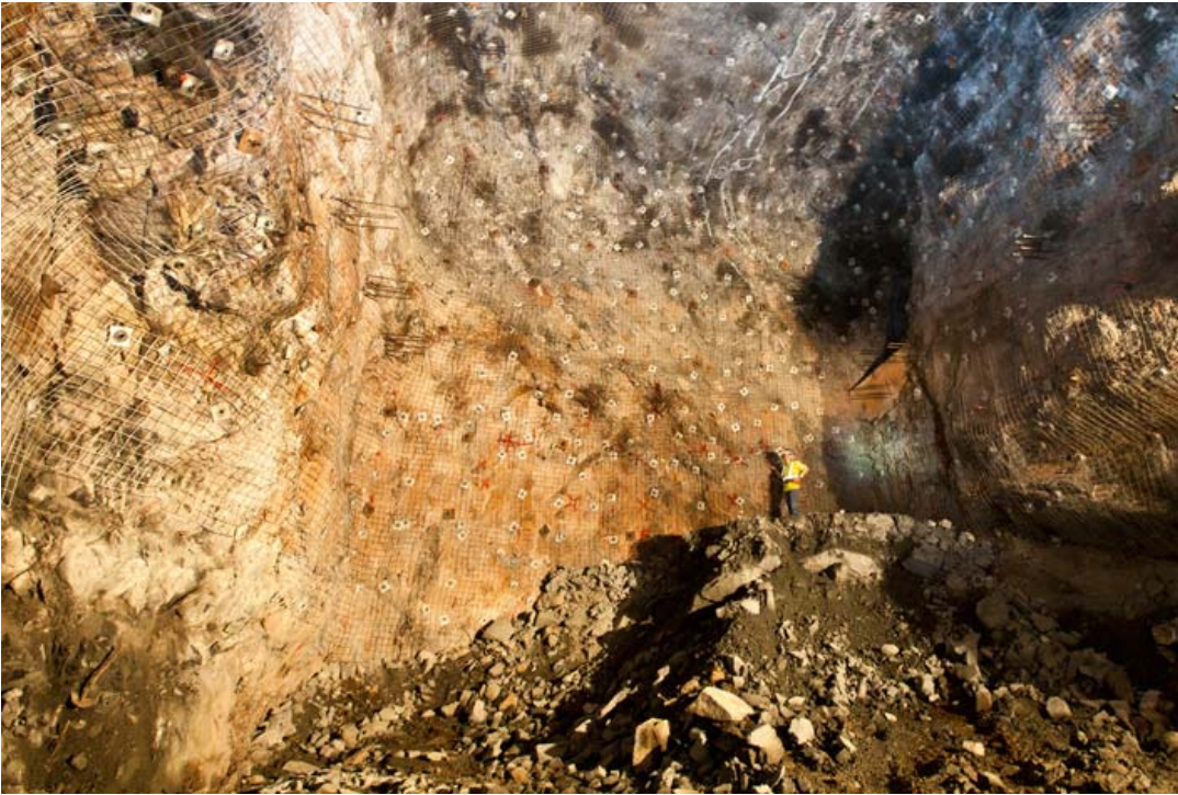
In July 2010, engineer Wendy Zawada stands on the last pile of rock that needed to be removed from the cavern for the LUX experiment, 4850 feet underground. Photo: Matt Kapust
