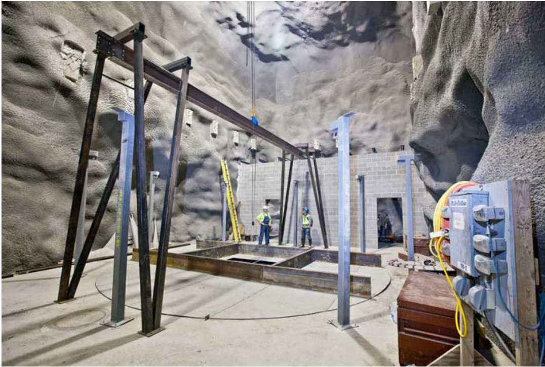
Construction workers built the water tank starting from the top. A temporary gantry was used to lift the lid off the ground, and welders attached the cylindrical walls below the lid, one ring at a time. Photo: Matt Kapust
