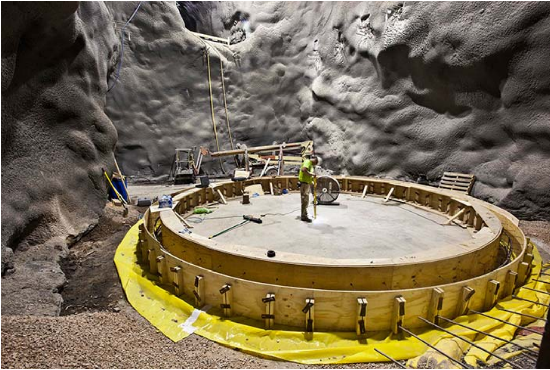
The floor of the Davis cavern is designed to support the heavy, cylindrical water tank that will surround the LUX detector. Photo: Matt Kapust
