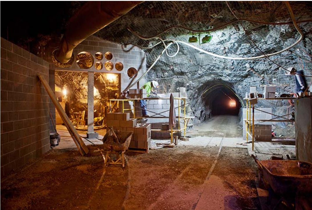
Construction workers are turning the former gold mine into a state-of-the-art underground research facility. The tunnel to the right provides secondary access to the Davis cavern, which will house the LUX experiment. The doorway to the left is the entrance to the Transition cavern, which will house the Majorana Demonstrator experiment and provide primary access to LUX. Photo: Matt Kapust
