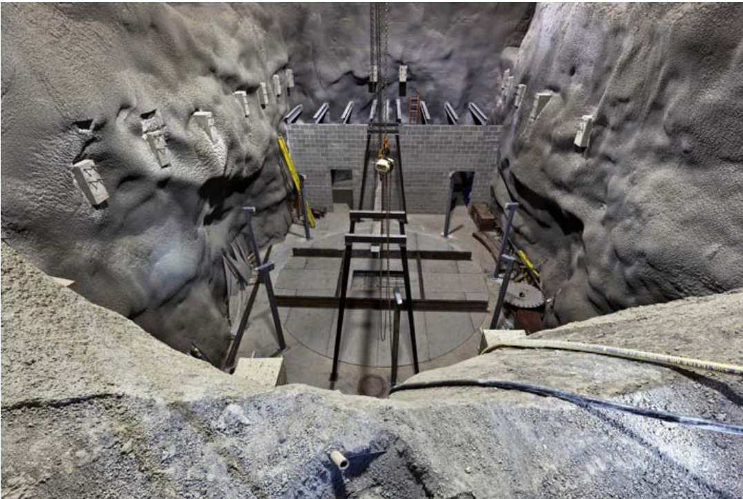
The LUX detector hall is ready for the installation of the large water tank. The lid of the tank, assembled from stainless steel plates, lies on the concrete floor. Photo: Matt Kapust
